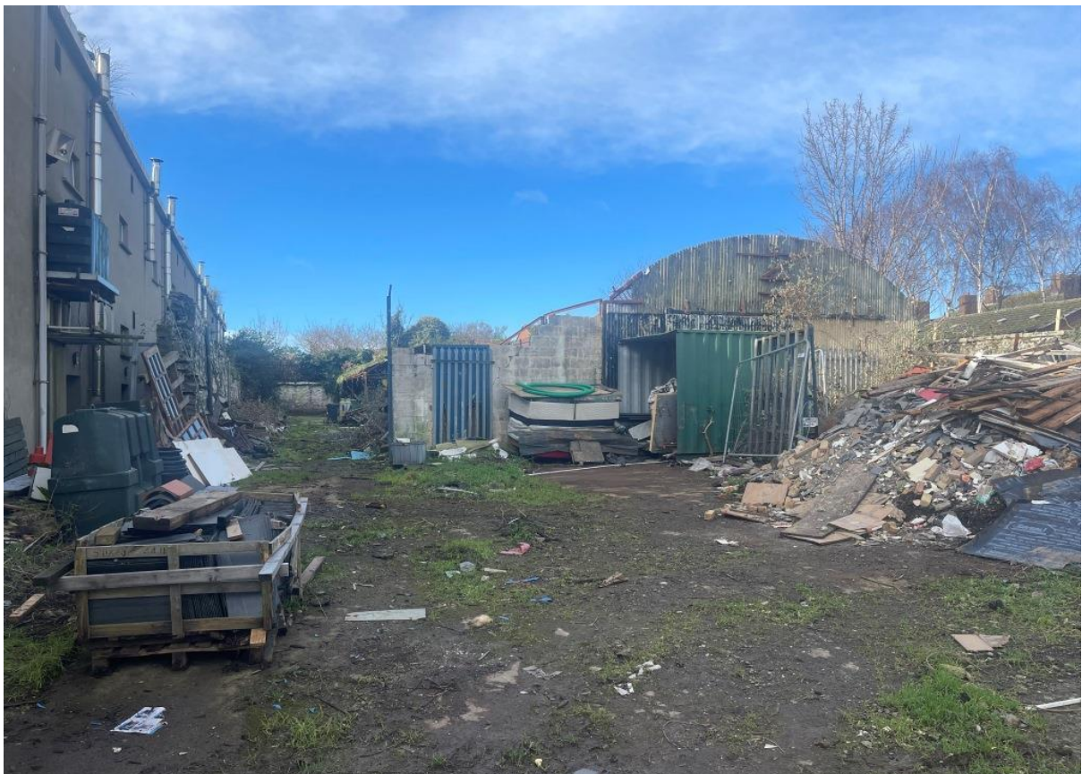
Plate 4: Remains of sheds within the northern portion of the development site – note the rear elevation of the modern industrial units on the left hand side of the photograph
